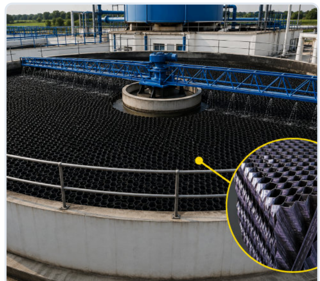
Fixed-Film Biological Reactor Installation
